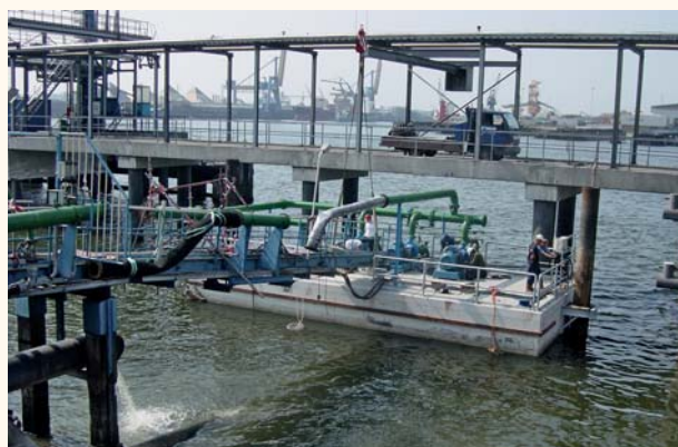
Pompstation in Botlek.
